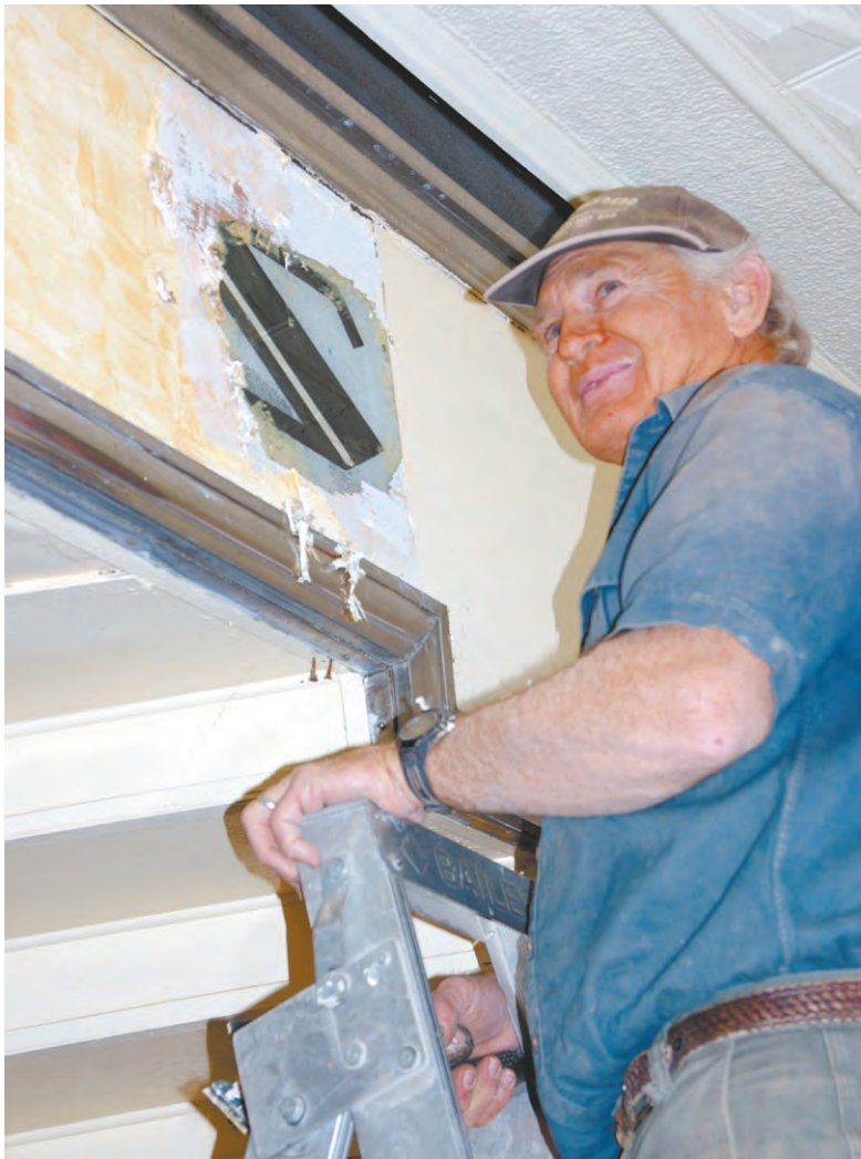
Doug Dunlop of Domenico Blu Building revealing the etched glass in May 2010
